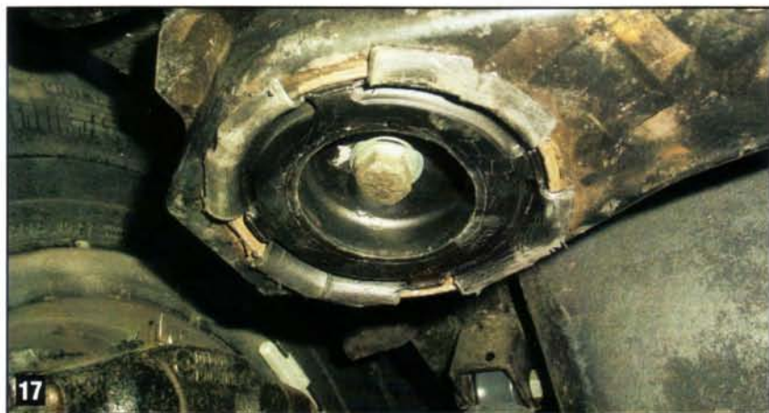
17 The crossmember and new bushings back in place, through-bolts torqued, ready for another 40 years and 90,000 miles.
